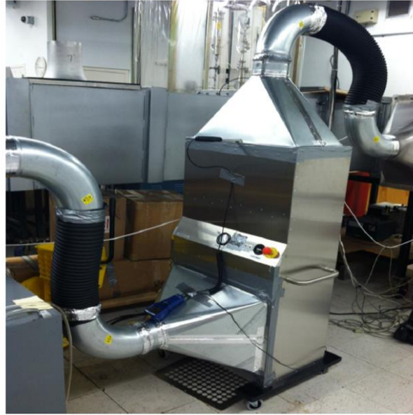
Figure 2. View of the ESP unit installed in the test duct. Air flow in the test duct is from left to right.
